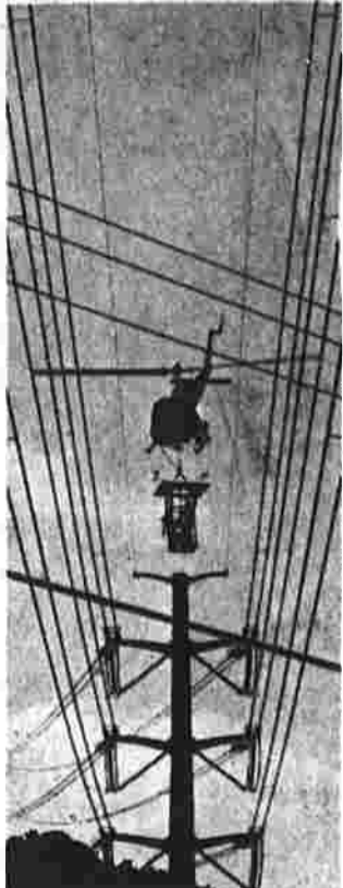
BIG LIFT for communications is provided by a helicopter depositing a newly developed portable servicing platform atop a transmission tower at Pomona, N.Y. Called the Decal Landing Deck Air Scaffold, it permits a maintenance man to transfer from the helicopter for rapid servicing of the tower.
